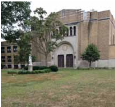
Removed concrete circle drive on Mull Avenue to help with water mitigation
